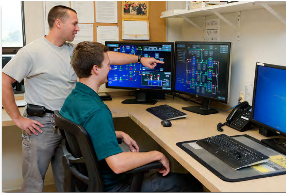
City public works staff monitor real-time information about the operation of the raw water treatment facility
