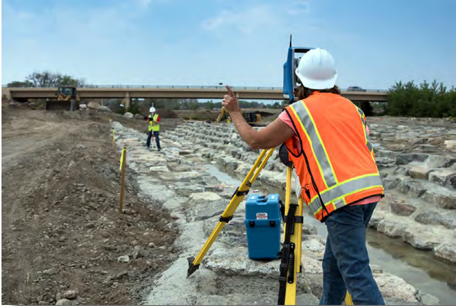
City surveyors work at the site of Dickens Farm Nature Area, scheduled to open in 2018
