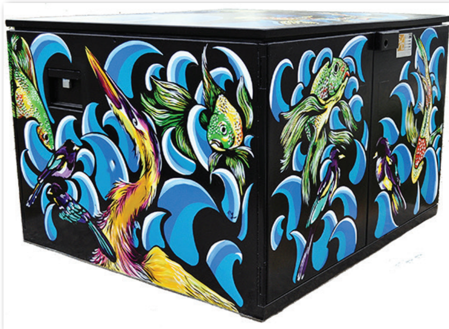
Longmont's Art in Public Places Program manages more than 80 permanent and temporary works of art, including "Shock Art" switchgear boxes throughout the city
