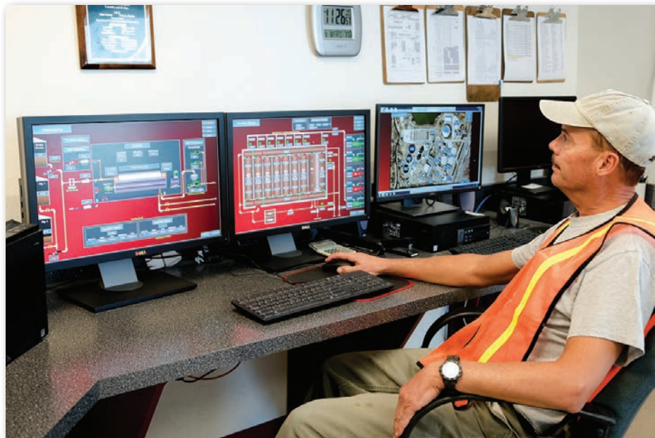
The Longmont Wastewater Treatment Plant is rated to treat up to 17 million gallons per day
