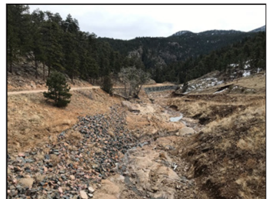
Figure 77. Looking east at the gabion wall that was constructed after the 2013 flood to prevent future erosion of Fire Road 1.
