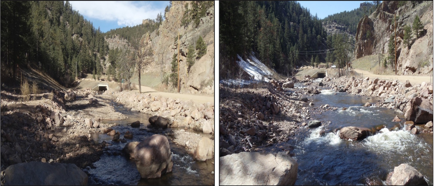
Figure 69. Phase 1: Restoration before and after: Looking upstream from main parking toward the box culvert in the distance. Left photo was taken in March, 2016, right photo of restoration was taken March, 2017.
