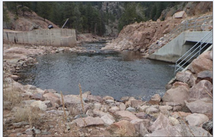
Figure 35. Concrete box culvert under road and Chimney Rock Dam (Photo DSSV08, RiverRestoration, 2019).
