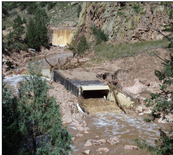
Figure 65. Ralph Price Reservoir (left) with log jam on Sept. 16, 2013 (CDWR, 2014). Damaged bridge culvert (right) below Longmont Dam.
