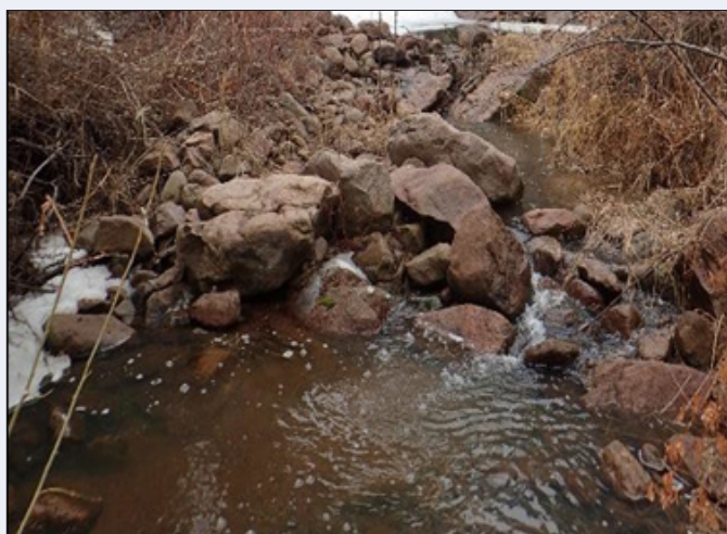
Figure 37. A shallow pool with cobble and boulder serving as grade controls (Photo LG08, RiverRestoration, 2019).
