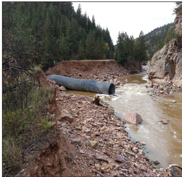
Figure 64. Button Rock Dam spillway (left) on Sept. 13, 2013 with near peak flows of over 10,000 cfs (CDWR, 2014). What remained of Longmont Dam Road (right) after the flood surge in the Preserve.
